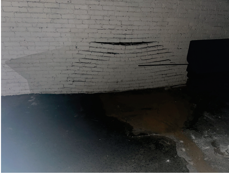
Depression and brick displacement in central portion of building
