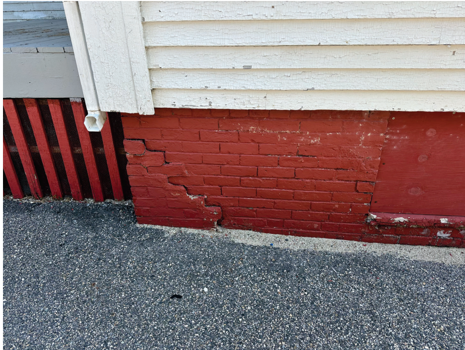
Brick displacement along Southeast perimeter wall
