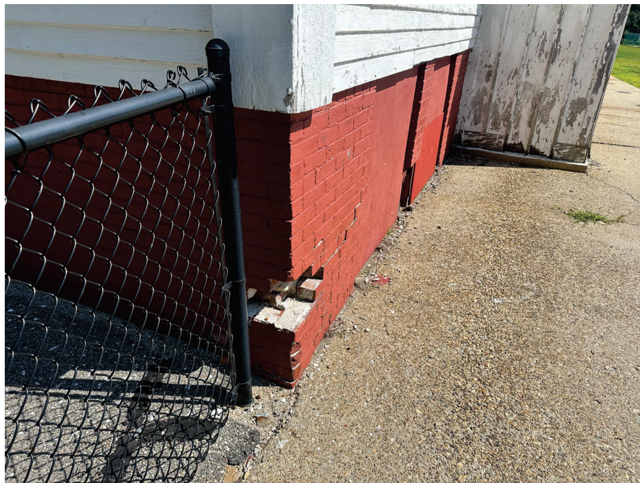
Missing brick on Southern building corner
