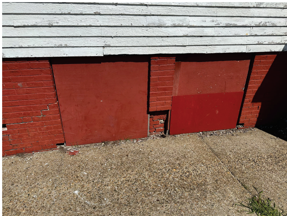
Missing brick and brick displacement along Southeast perimeter wall
